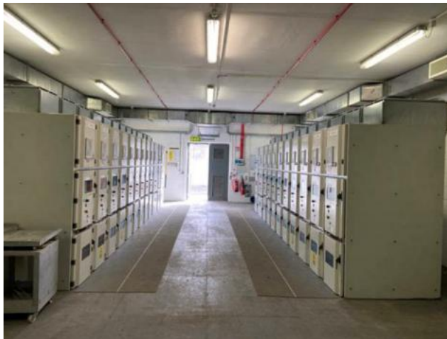
Figure 6.12: CIP27.04.15 – Airport Existing MV Network Upgrades – Example of Modern MV Switchgear
