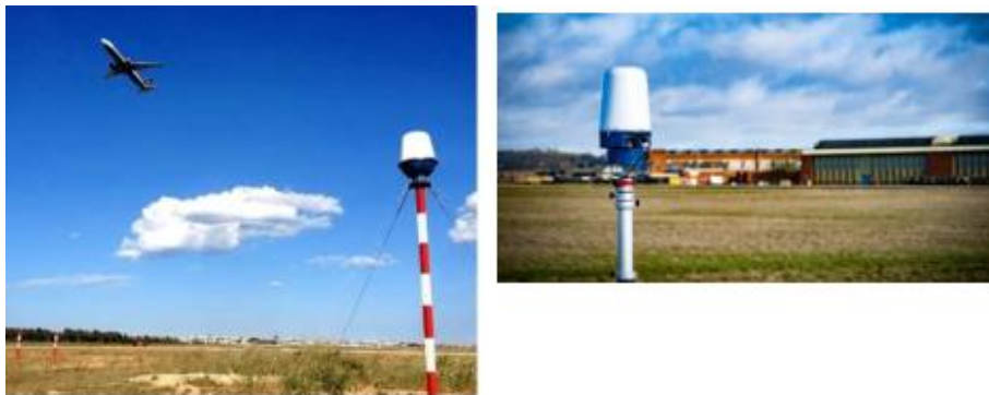
Figure 7.1: Example of radar intrusion detection system installation
