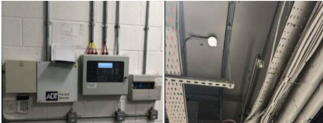
Figure 6.19: Existing Life Safety Systems and Controls
