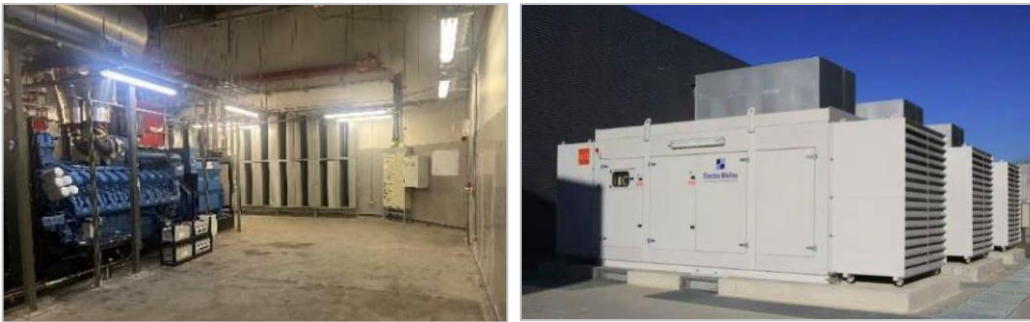
Figure 6.14: CIP27.04.17 Primary Standby Power Generation Upgrade – Terminal 2 Generator Room and Typical Prime Generator Site
