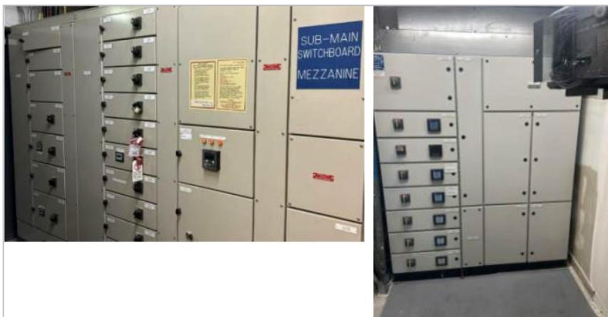
Figure 6.13: CIP27.04.16 Terminals and Piers Low Voltage (LV) Electrical Upgrade - LV Sub Mains Distribution Boards
