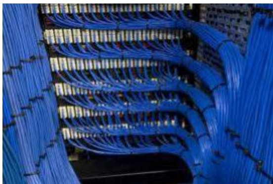
Figure 8.8: Network Data Cabling
