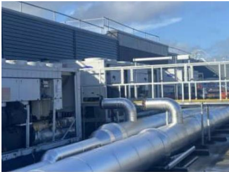
Figure 6.20: Example Chiller Replacements in 2021
