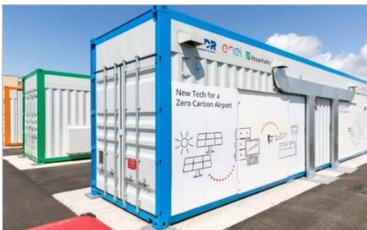
Figure 3.4: CIP27.01.03 – Solar PV and Energy Storage - Battery Energy Rome Airport
