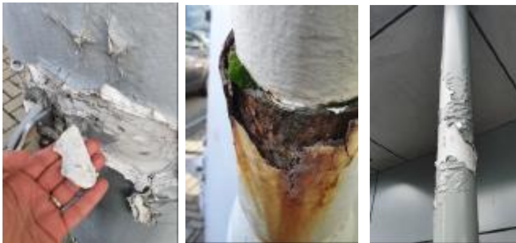
Figure 6.5: CIP27.04.04 – Building Fabric Upgrade – Deterioration of building elements
