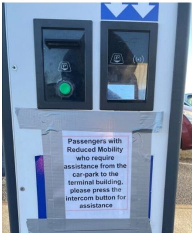
Figure 4: Assistance Call Button at Barrier to Car Park
