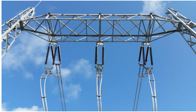
Figure 5.2: Second Medium Voltage (MV) Connection Point
