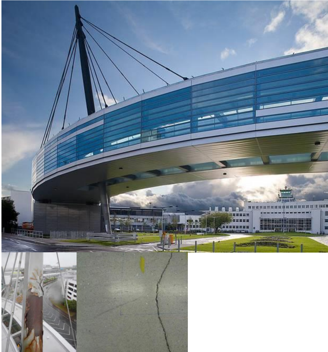
Figure 4.18: Skybridge Rehabilitation - Skybridge at Dublin Airport / Corrosion at Steel Structure / Cracks in Terrazzo Floor
