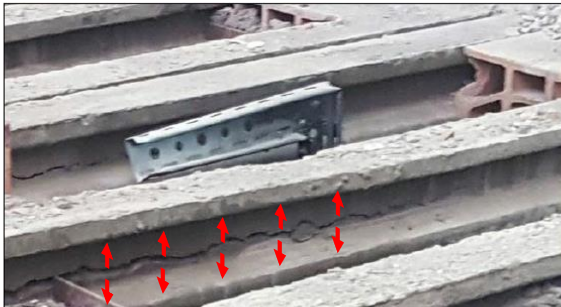
FIGURE 7.2 STRUCTURAL BEAM CRACKING & PASSENGER PROXIMITY TO POTENTIAL FAILURE
