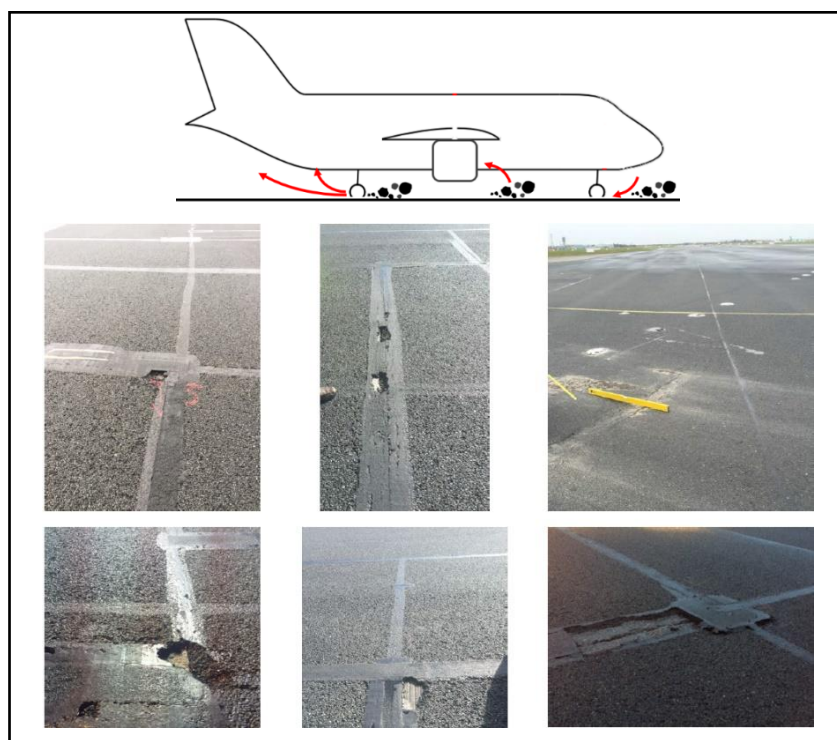
FIGURE 7.3 CRITICAL OVERLAY FAILURE
