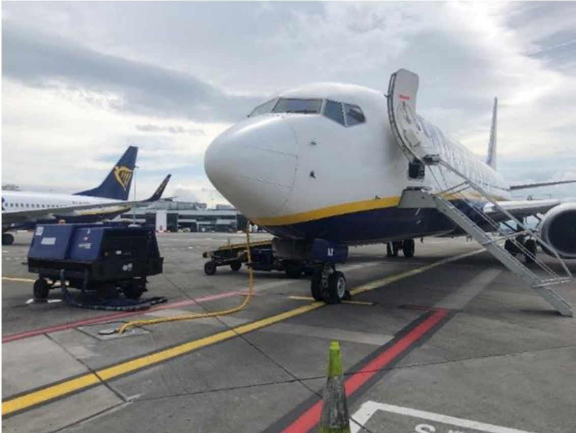
Figure 7.6: Fixed Electrical Ground Power Phase 3
