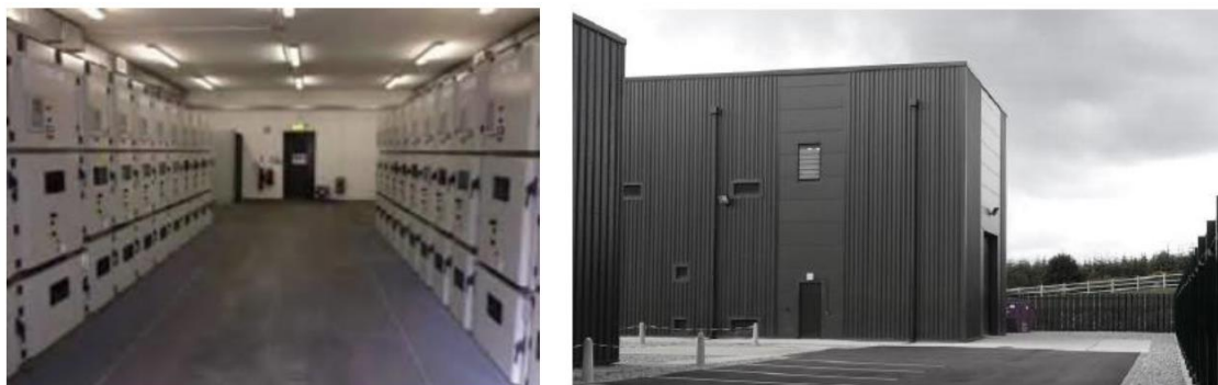
Figure 4.2: MV Resilience Substation
