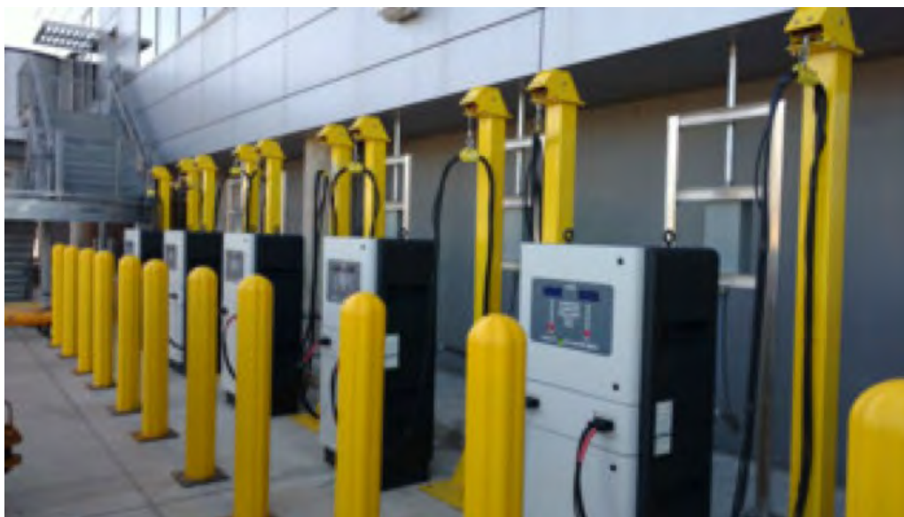
Exhibit 1. Example of outdoor GSE fast charging equipment
