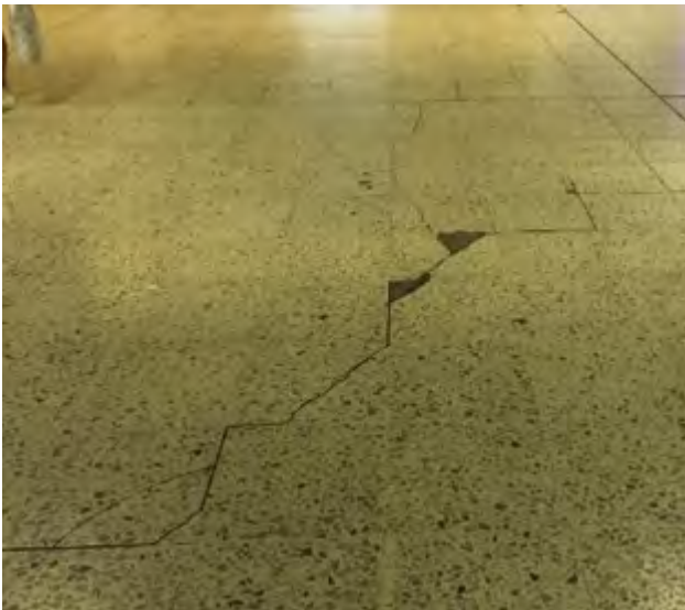
Exhibit 3. Existing baggage reclaim hall condition of floor
