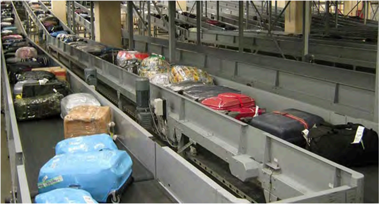
Exhibit 2. Photograph of an EBS system - Typical
