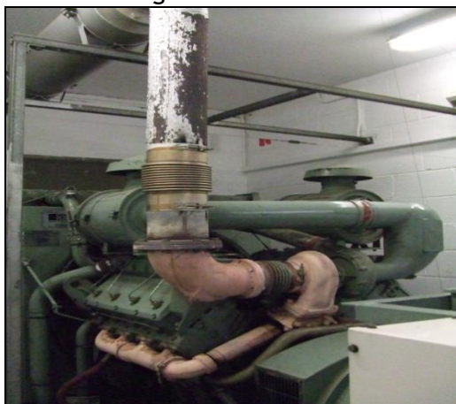
Existing Airfield Generator
